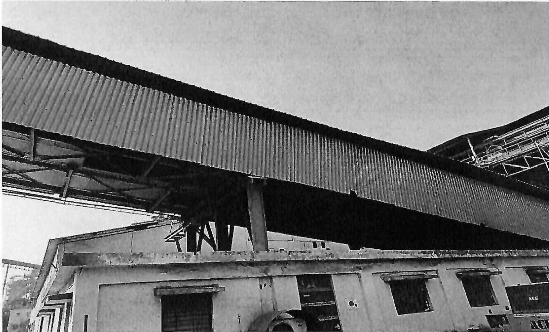
Fig.1. Closed Belt Conveyor
