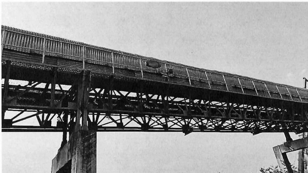
Fig.2. Closed Belt Conveyor
